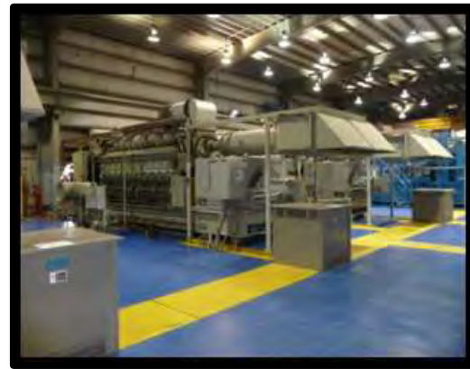
Photo 3.14-1. Power Generation Facility
