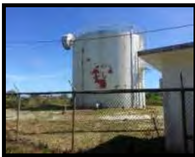
Photo 3.14-5. Marpo Water Storage Tank (250,000 Gallon Tank)
